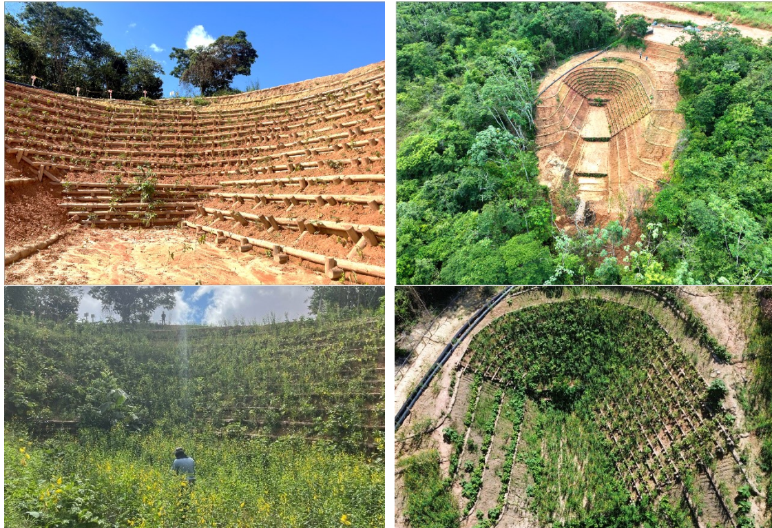
Figure 11. General aspect of the soil bioengineering project at the conclusion phase on 03/05/24 (above) and 15/07/2024 (under).
