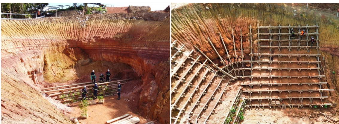
Figure 10. Execution of the activities of the double living support wall live wooden cribwall on 18/01/24 (left) and the live slope grid on 14/03/24 (right).
